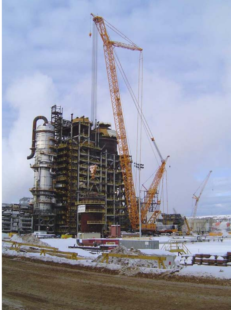
Figure 10: Terex-Demag CC 8800 Mobile crane involved in lifting work at a chemical refinery. (Photo courtesy Hans-Peter Franzen, Terex-Demag).
